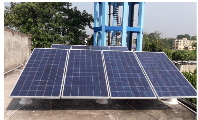
10 KWP ON-GRID SOLAR POWER PLANT BDO OFFICE, JALANGI, MURSHIDABAD
