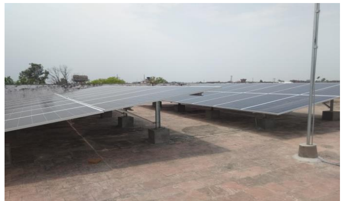
40 KWP ON-GRID SOLAR POWER PLANT CIVIL COURT NAWADA, BIHAR
