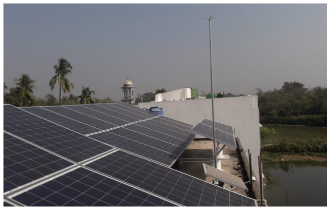
10 KWP ON-GRID SOLAR POWER PLANT GRAM PANCHAYAT OFFICE JURANPUR, MURSHIDABAD
