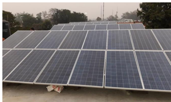
30 KWP ON-GRID SOLAR POWER PLANT SOUTH EASTERN RAILWAY, ADRA DIVISION, WEST BENGAL
