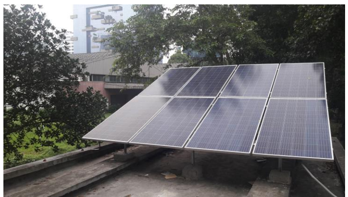
5.2 KWP OFF-GRID SOLAR POWER PLANT SALT LAKE, KOLKATA, SIEMENS LIMITED
