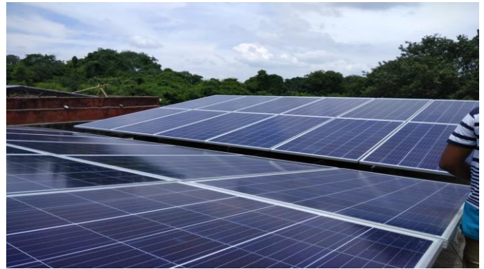
90 KWP SOLAR POWER PLANT CENTRAL JAIL, GAYA, BIHAR
