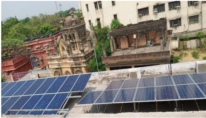
12 KWP SOLAR POWER PLANT DRDA, GAYA, BIHAR
