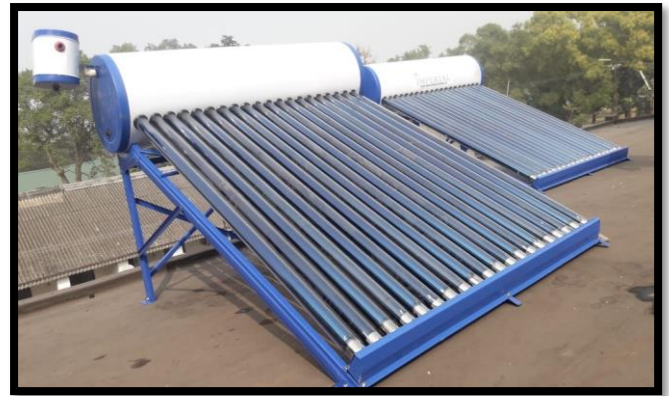
800 LPD ETC SYSTEM ADRA ARMY CAMP, PURULIA, W.B.
