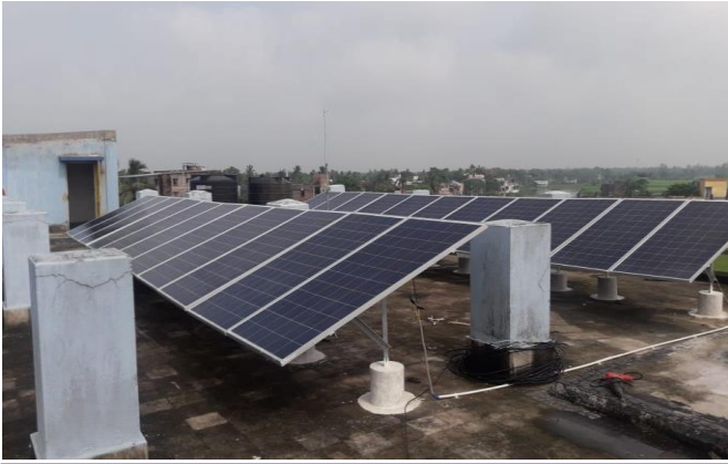
7 KWP ON-GRID SOLAR POWER PLANT SDO OFFICE, DOMKAL, MURSHIDABAD
