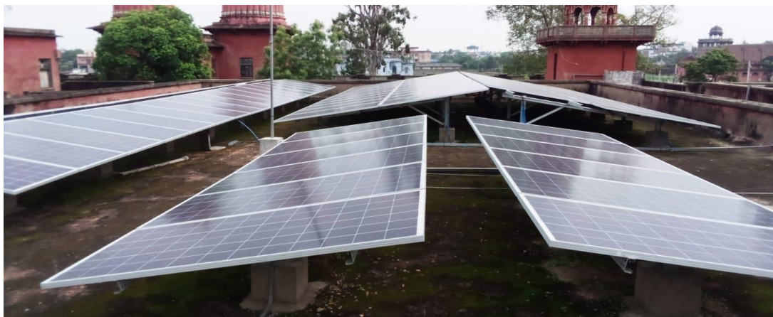
225 KW ON-GRID SOLAR POWER PLANT LALIT NARAYAN MITHILA UNIVERSITY DARBHANGA, BIHAR
