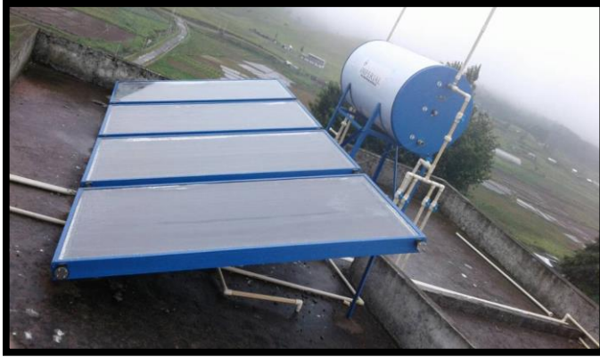
500 LPD, HOLY CROSS HEALTH CENTRE, MAIRANG, SHILLONG
