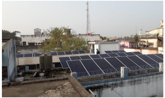
10 KWP ON-GRID SOLAR POWER PLANT GRAM PANCHAYAT OFFICE ISLAMPUR CHOWK, MURSHIDABAD
