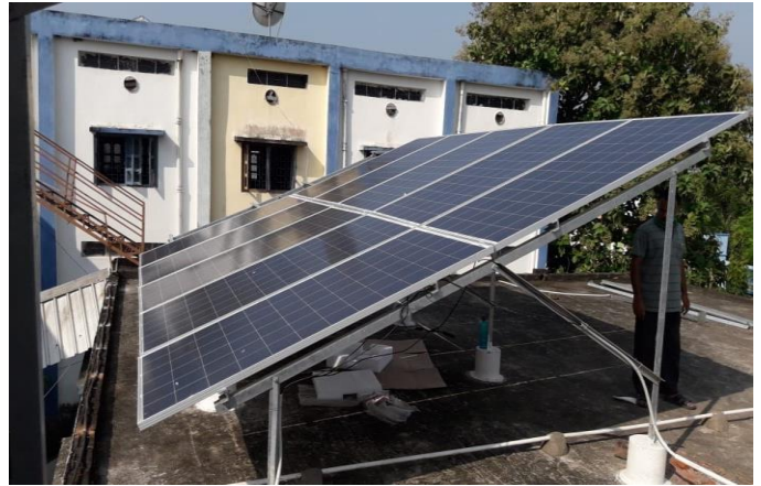
10 KWP ON-GRID SOLAR POWER PLANT GRAM PANCHAYAT OFFICE DHULAUARI, MURSHIDABAD
