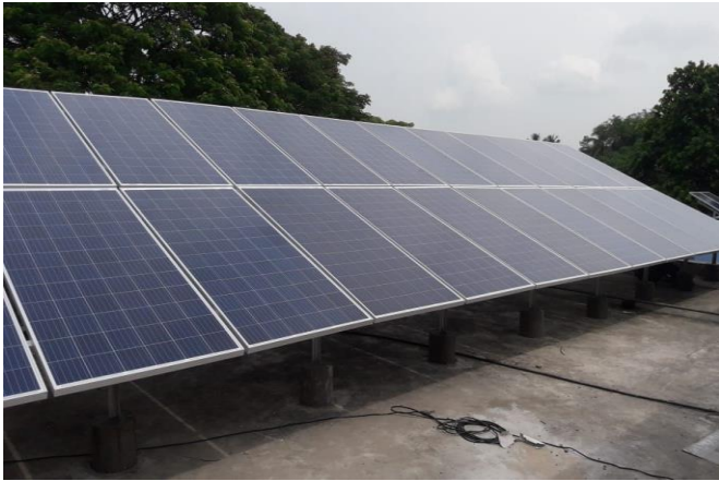
30 KWP ON-GRID SOLAR POWER PLANT BDO OFFICE, RANINAGAR-I, MURSHIDABAD
