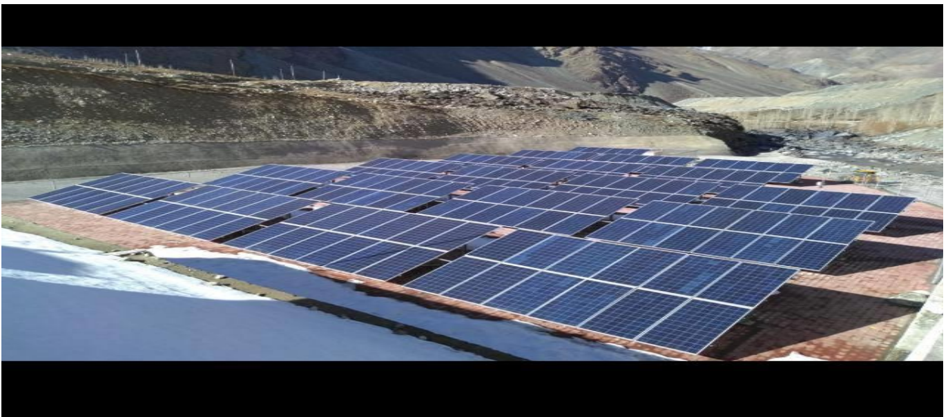
65 KWP OFF-GRID SOLAR POWER PLANT – NHPC KARGIL
