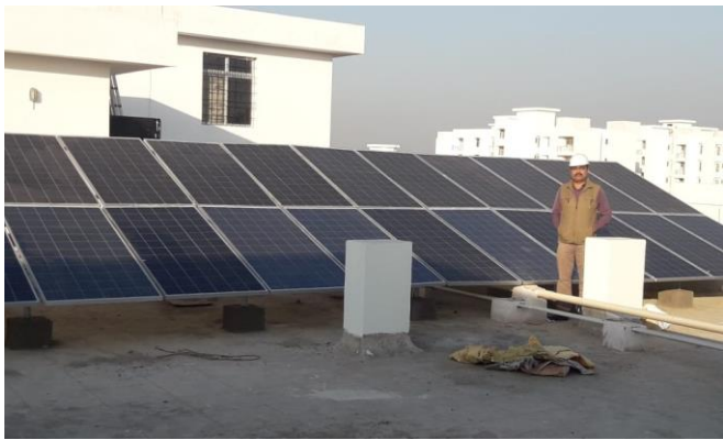
13 KWP OFF-GRID SOLAR POWER PLANT SCIENCE & TECHNICAL UNIVERSITY, NAMKOM, RANCHI, JHARKHAND
